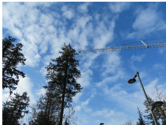
The crane on Lot 11 comes close to the edge of the furthest east tree in the vegetative buffer around the nest.
